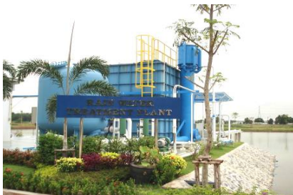
Rain water treatment plant
