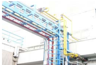
Natural Gas Pipe
