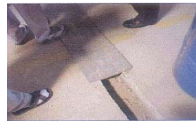
channel to limit chemical leak area
